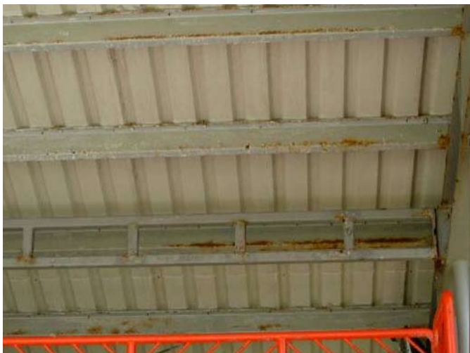
CORROSION ON UNDERSIDE OF CORRUGATED SHEETS
